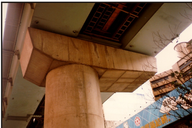
Cracked concrete pier in Taiwan
