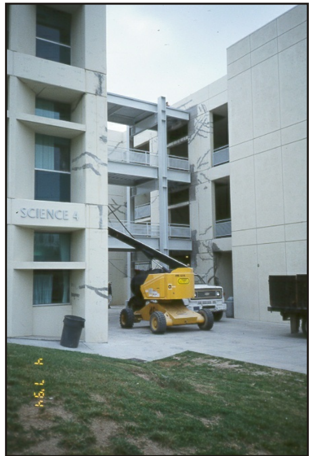
Extensive cracking due to earthquake damage
