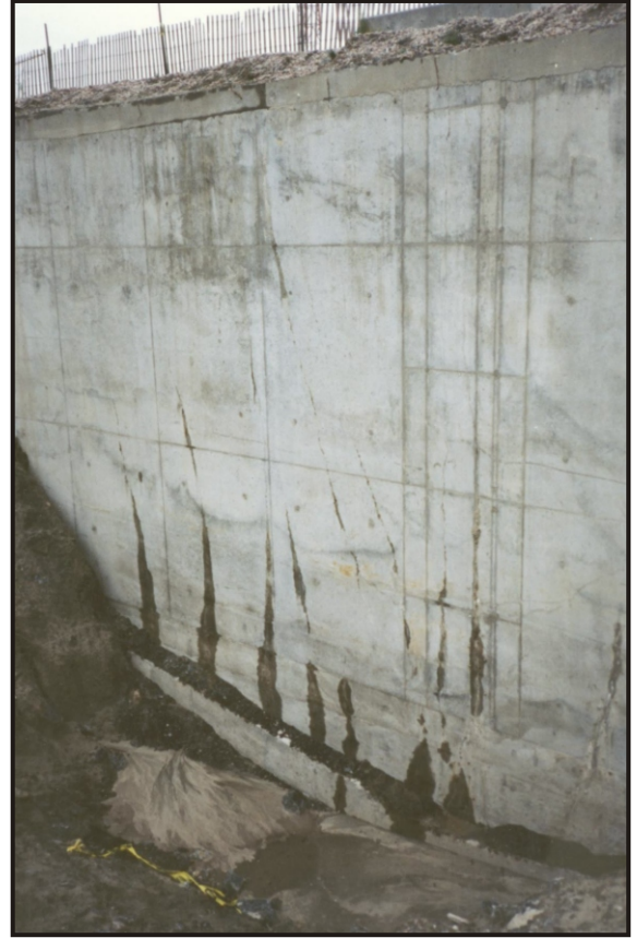
Water leakage through cracks in walls
