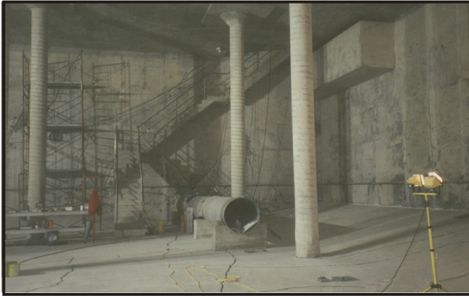
View inside a typical 10 million gallon reservoir
